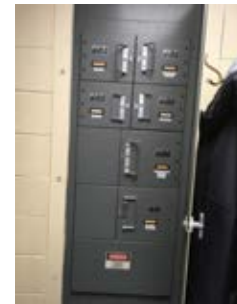
Main Electric Service
