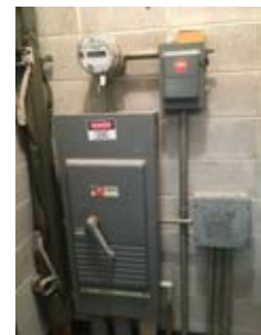
Main Switchboard & Meter
