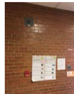
Rudimentary Fire Alarm Devices
