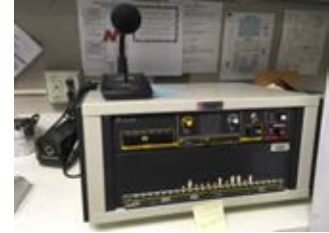
Existing Intercom Head-End
